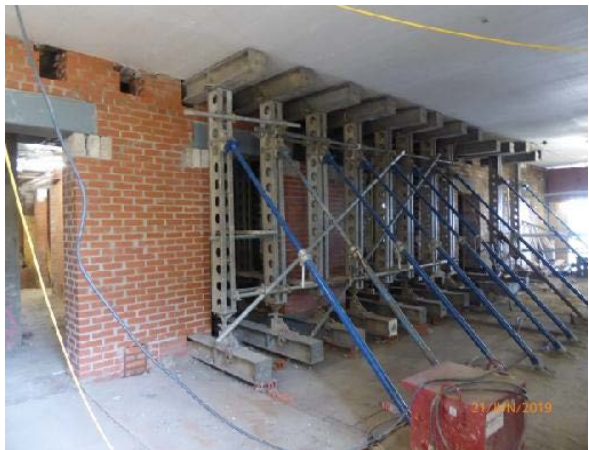
Looking East: Temporary propping in place for formation of the new door openings to the passenger lift and Staff circulation corridor from the main entrance lobby.
