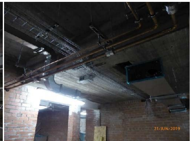
Circulation/Utility Space/Staircase to undercroft structural openings – Electrical wiring insitu.
