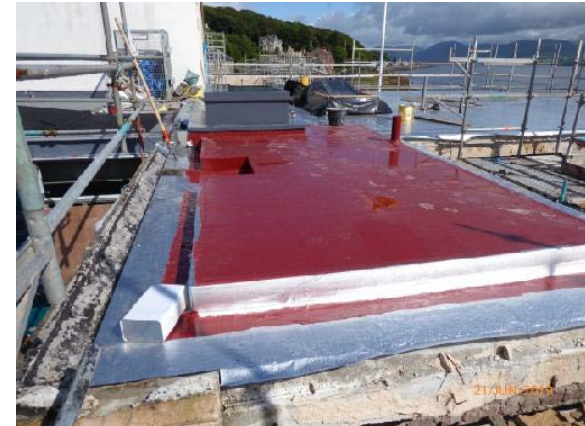
Looking North: General View – Roof over stairwell 1 (Adj. Exhibition/Function suite) NB: insulation insitu and roof basecoat (red) in progress.
