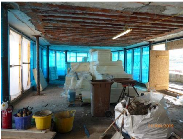
General View of the Exhibition / Function area (the insulation materials stored on the floor are for the Canopy roof above).
